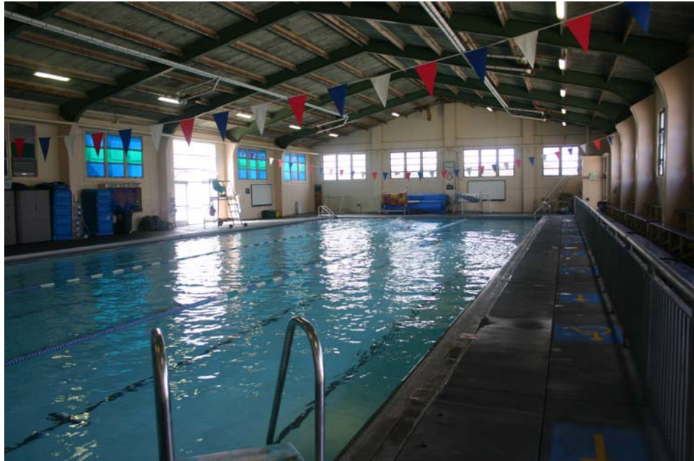
Exhibit 10: Pool Deck Standing Water
