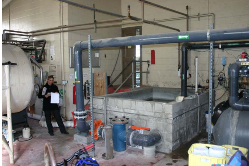
Existing Surge Pit Leaking
